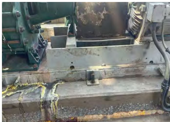
ACID GUARD® 135 Pump Base showing acid exposure
