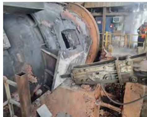
Anode Furnace Mouth lined with ARMORMAX®
