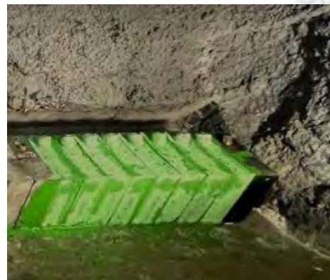
Tuyere System installed with Peirce-Smith Converter
