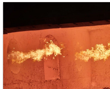
Burner wall 6 months of service
