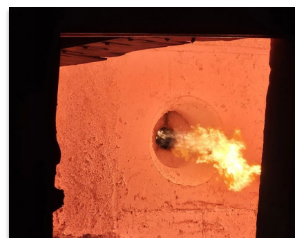
Burner wall 6 months of service
