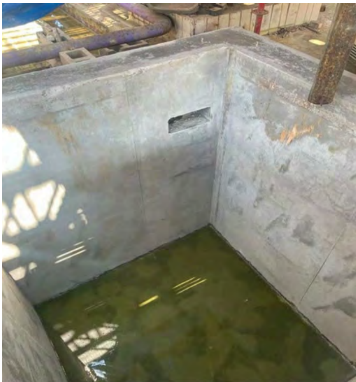
ACID GUARD® PC in Acid Pond
