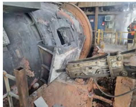
Anode Furnace Mouth lined with ARMORMAX®
