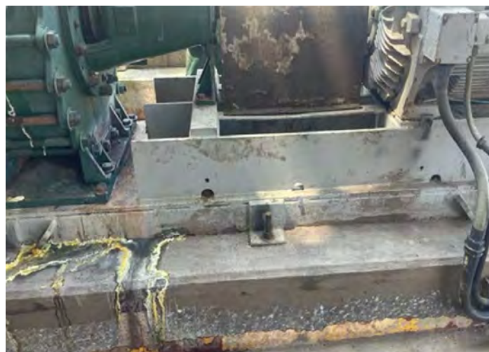
ACID GUARD® 135 Pump Base showing acid exposure
