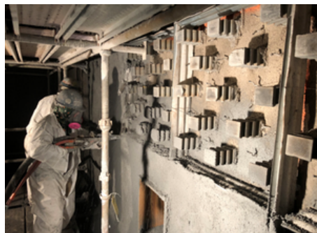
NANO-TEK® installation in a settling chamber.
