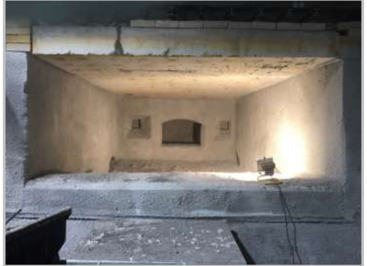
AFTER: QUICK-FIRE® 85 G installed
