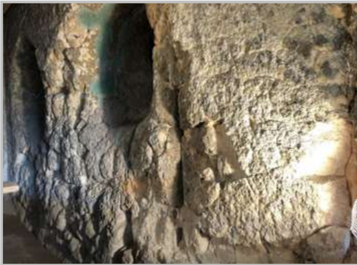
BEFORE: Furnace with material needing repair
