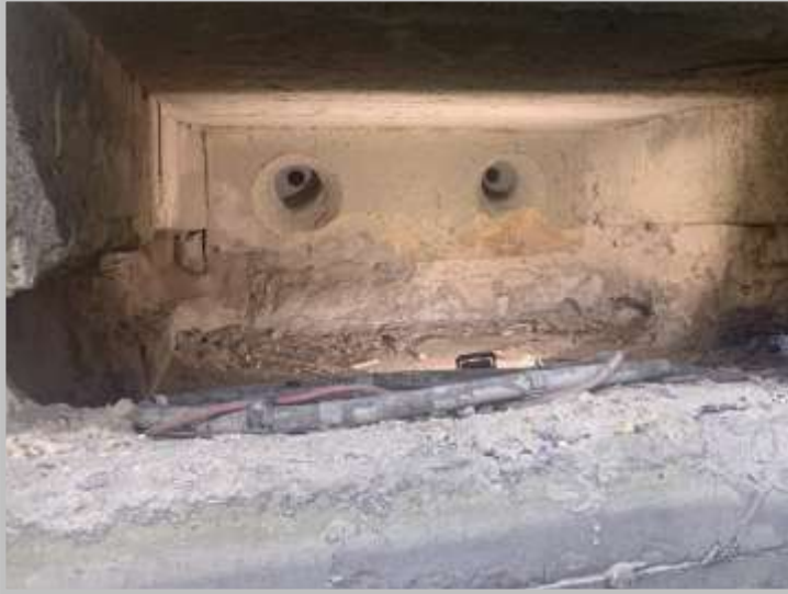
BEFORE: Furnace with material needing repair
