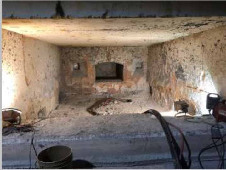
BEFORE: Furnace with material needing repair
