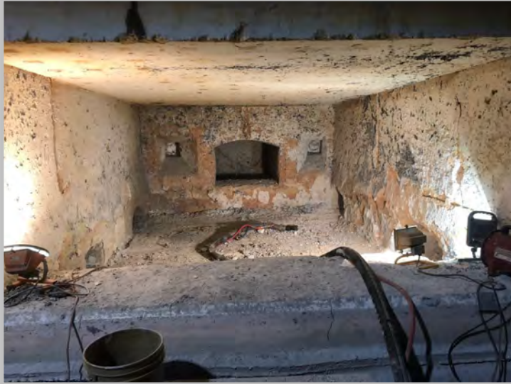
BEFORE: Furnace with material needing repair
