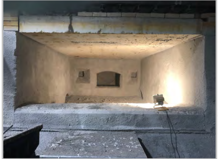
AFTER: QUICK-FIRE® 85 G installed
