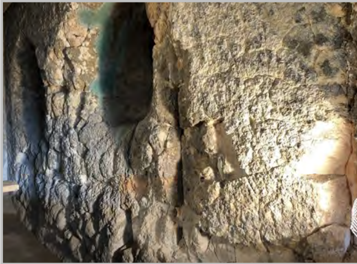
BEFORE: Furnace with material needing repair
