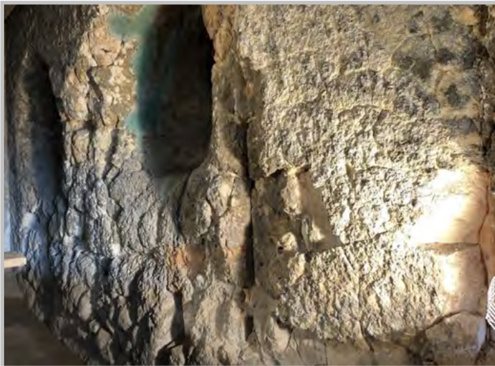
BEFORE: Furnace with material needing repair
