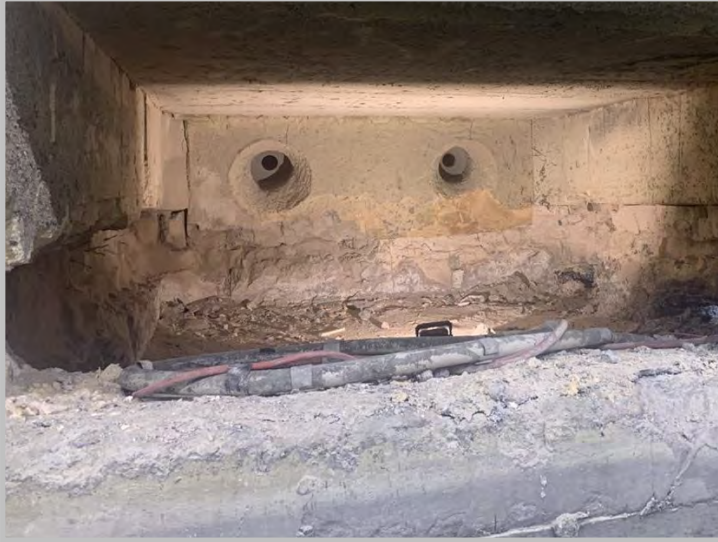
BEFORE: Furnace with material needing repair
