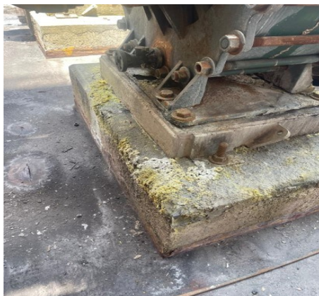
ACID GUARD™ 135 Pump Base after one year
