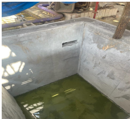
ACID GUARD™ PC Acid Pit
