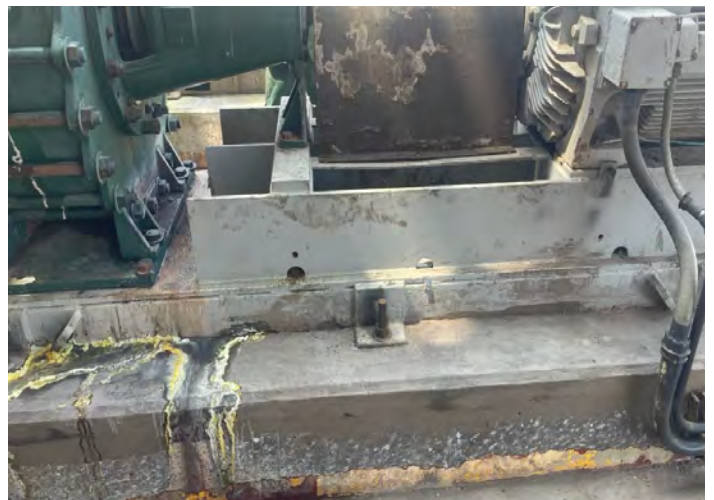
ACID GUARD 135 Pump Base showing acid exposure
