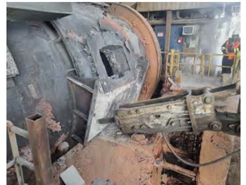
Anode Furnace Mouth lined with ARMORMAX®
