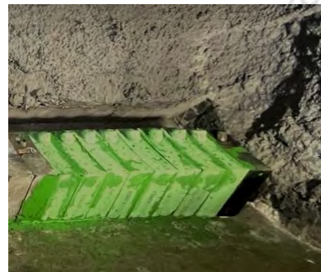
Tuyere System installed with Peirce-Smith Converter
