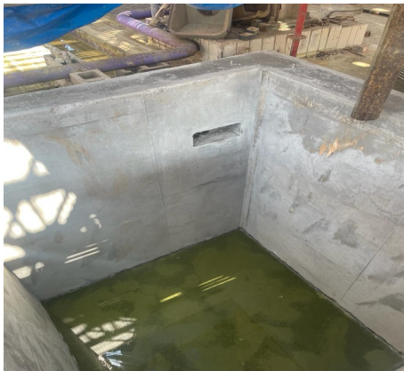
STACKLINE B PC Acid Pit
