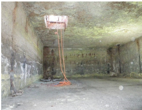
Sulfur Pit (Before)
