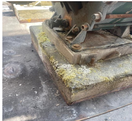
PG 135 Pump Base after one year
