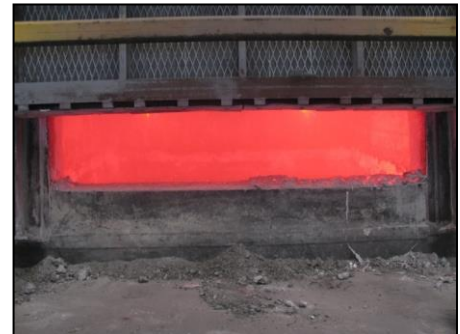
ARMORMAX® 70 AC sill after 10 months of service
