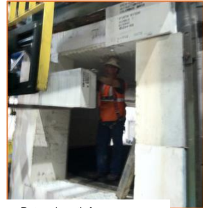
Rotary hearth furnace charge door lintel in service 2 years
