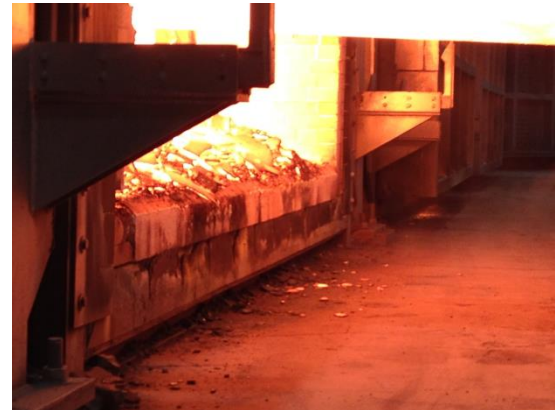
2450°F Forge furnace sill after 15 months in service
