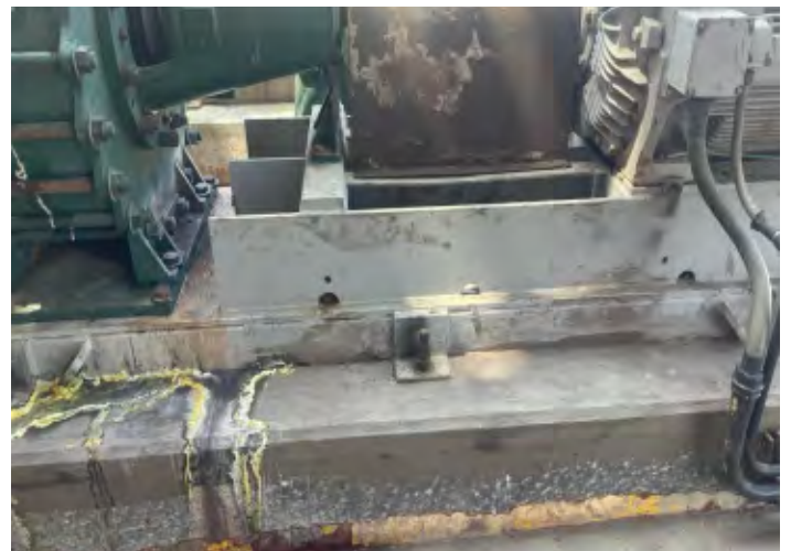
PG 135 Pump Base showing acid exposure
