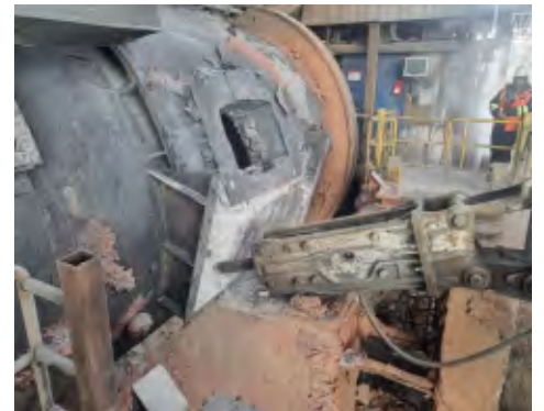
Anode Furnace Mouth lined with ARMORMAX ®
