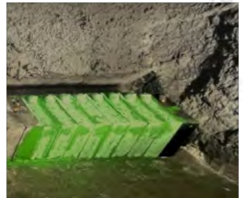
Tuyere System installed with Peirce-Smith Converter
