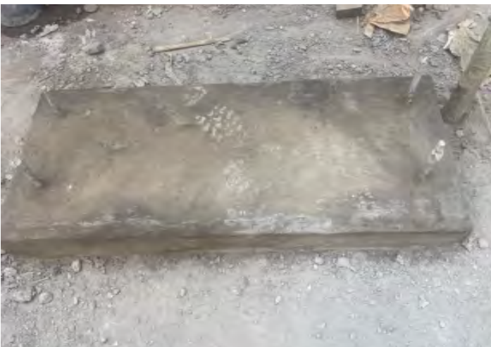
PG 135 Pump Base exposed to occasional acid contact
