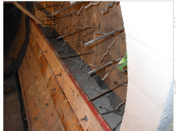
Rotary cooler with ARMORMAX® 70 SR
