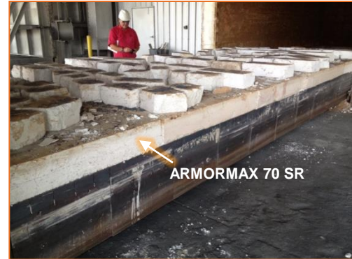
ARMORMAX 70 SR perimeter adjacent to competitive 60% alumina castable
