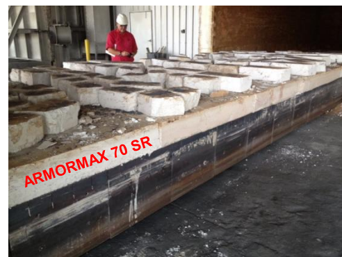
ARMORMAX 70 SR perimeter adjacent to competitive 70% alumina castable
